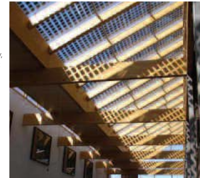
A photovoltaic array integrated onto the roof atrium of the student services building at Southampton University © University of Southampton
