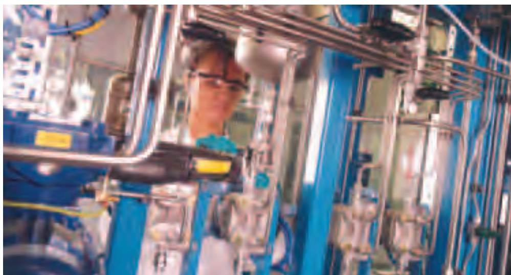
Mini-Plant for the development of the ethyl acetate production process © Davy Process Technology
