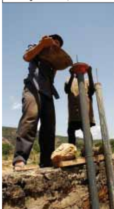
Joe Mulligan and a team member casting test piles for the river crossing © Anna Tompsett
