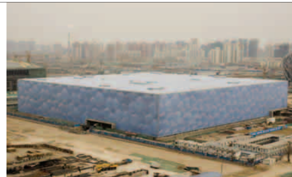
The Water Cube nearing completion. It will be the venue for the swimming, diving, synchronised swimming and the water polo competitions in August 2008 © Martin Saunders Photography
