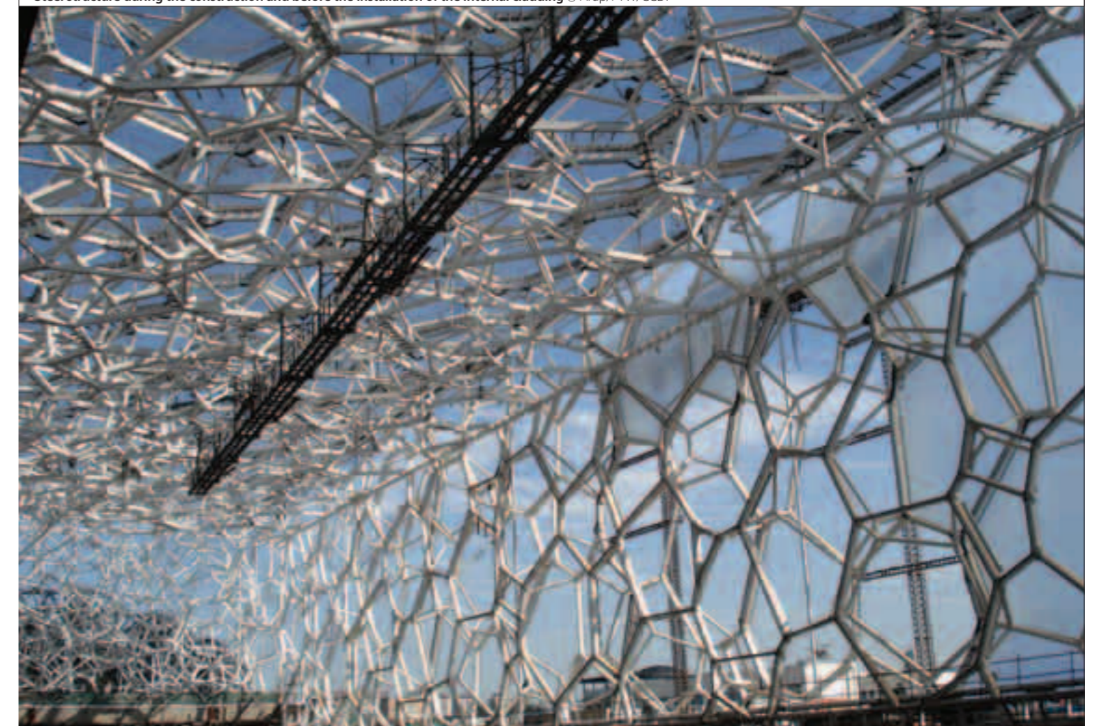
Steel structure during the construction and before the installation of the internal cladding © Arup/PTW/CCDI
