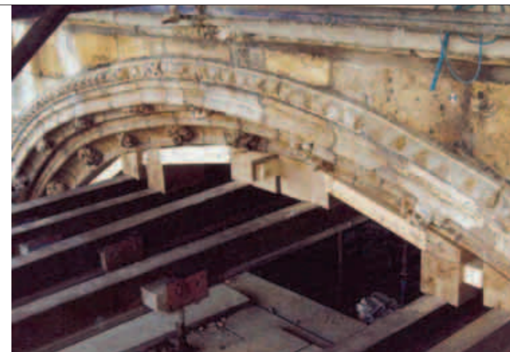
A view of the upper section of the arch with the tracery removed. The timber blocks were wedged up to the arch to keep it in place while lateral wedges were installed to stop the main wedges slipping. At any one time up to two of the steel support beams (needles) could be taken out to allow removal or installation of individual stones © Geoff Clifton
