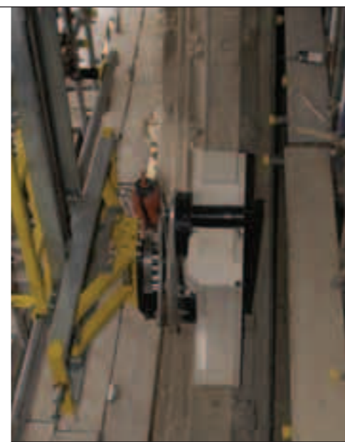
The stone handling device: the vertical grey bars are the rails on which the machine moves up and down, these are themselves attached to two horizontal bars which are attached to the structural scaffold, allowing the machine to traverse the whole window. Through this, individual stones can be aligned exactly in the right position, despite the distorted geometry of the tracery © Geoff Clifton
