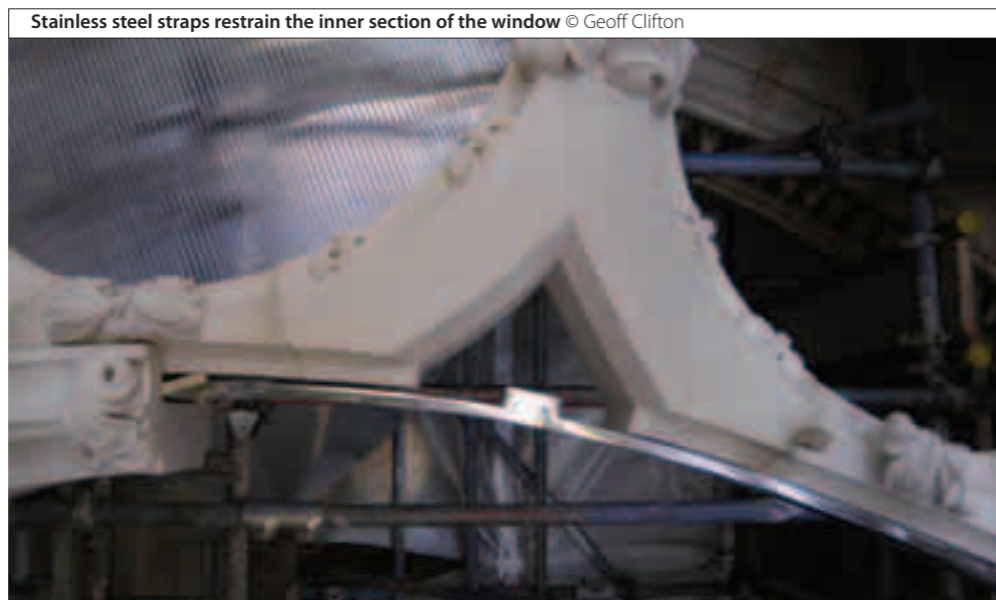
Stainless steel straps restrain the inner section of the window © Geoff Clifton
