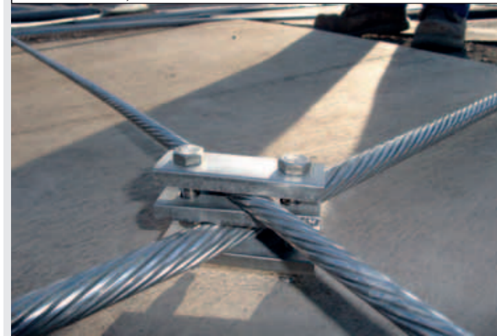
There are over 3,000 stainless steel cable clamps that connect the cables on Temenos © Freyssinet
