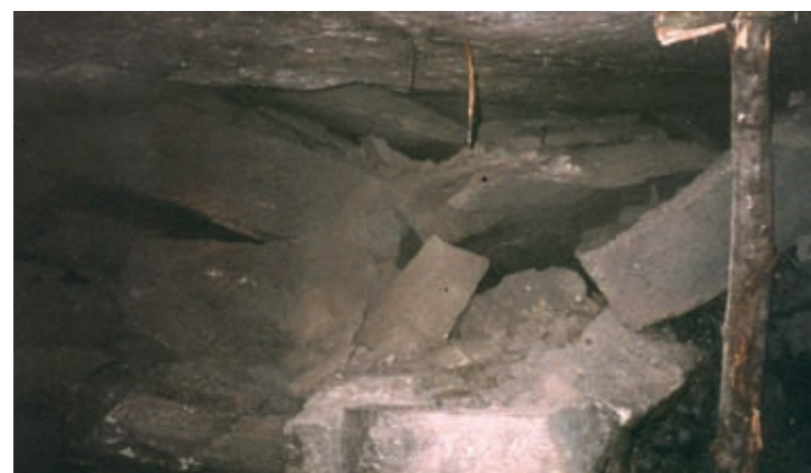
A rare photo showing the formation of goaf after total extraction of a coal seam using longwall methods (Hlobane Colliery, South Africa) © Paul Younger
