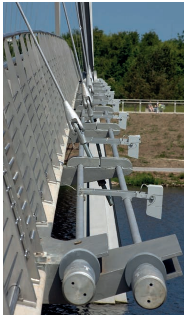
Pairs of longitudinal cables run either side of the deck units. These act as ties to the arch whilst also compressing the deck units together © Morley von Sternberg
