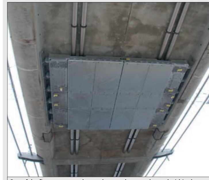
One of the five-tonne tuned mass dampers hung under, and within the profile of the deck of the Infinity Footbridge © Tim Harris, Expedition
