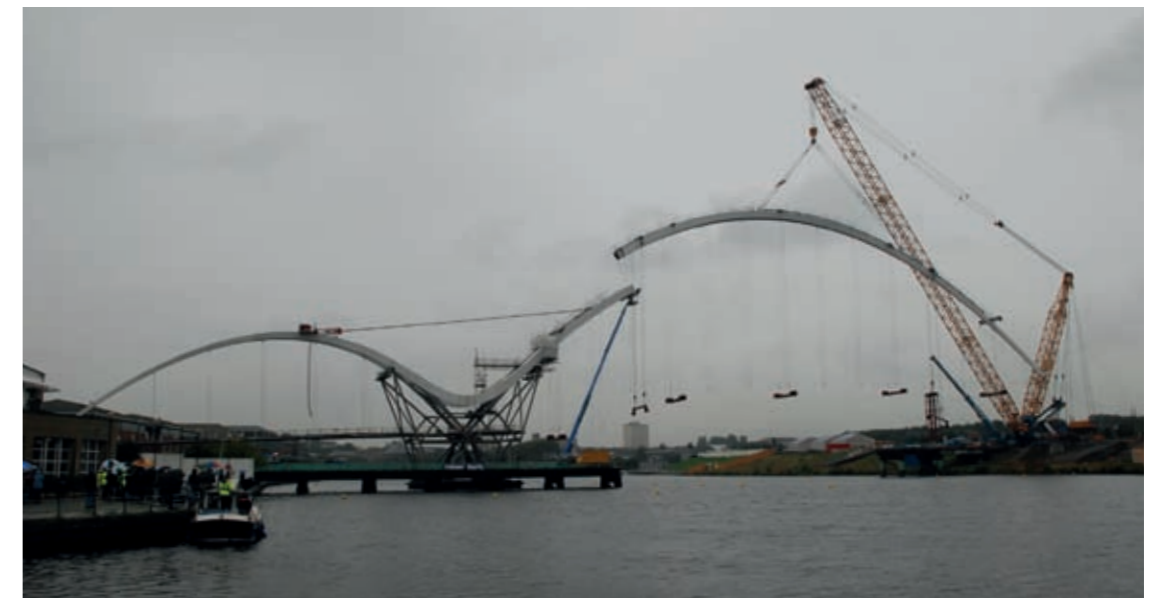
The north arch was lifted into place on one of the wettest days of construction. Hundreds of people came to watch the 1,500 tonne mobile crane lift the arch into place © Tim Harris, Expedition
