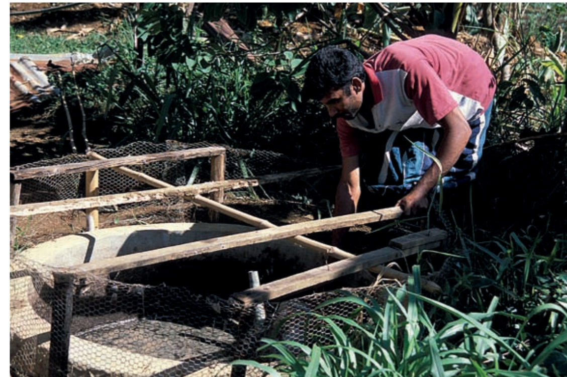
An input tank of a biogas digester being installed in Sri Lanka. The resultant biogas provides a clean cooking and lighting fuel that can be produced on a scale varying from a small household system to a large commercial plant of several thousand cubic metres.
