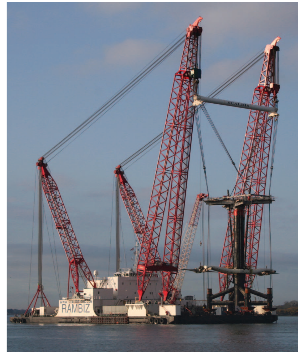
The Rambiz heavy lift crane-barge (lifting capacity over 3,000 tonnes) which delivered the 1,000 tonne SeaGen prototype to its site in Strangford Narrows in April 2008. SeaGen, fitted with its temporary drilling platform at the top of its structure, can be seen suspended below the crane jibs. The four-legged jacket which stands on the seabed is also visible
