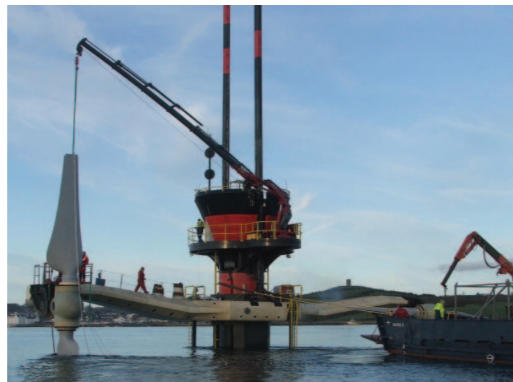
SeaGen with its cross-arm and twin rotors raised out of the water to allow access for maintenance from a small boat. In this instance, the engineers are replacing a rotor blade: a relatively straightforward operation using the boat's onboard finger crane and a small service vessel to deliver the 1.5 tonne blade
