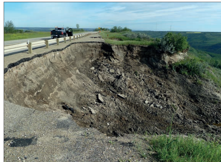
Landslide damage to a highway in Peace River, Alberta, Canada © Alister Smith
