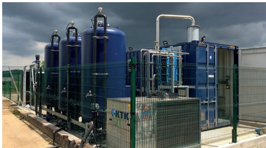
Cornelsen's remediation plant, which uses separation approaches © Cornelsen Ltd
