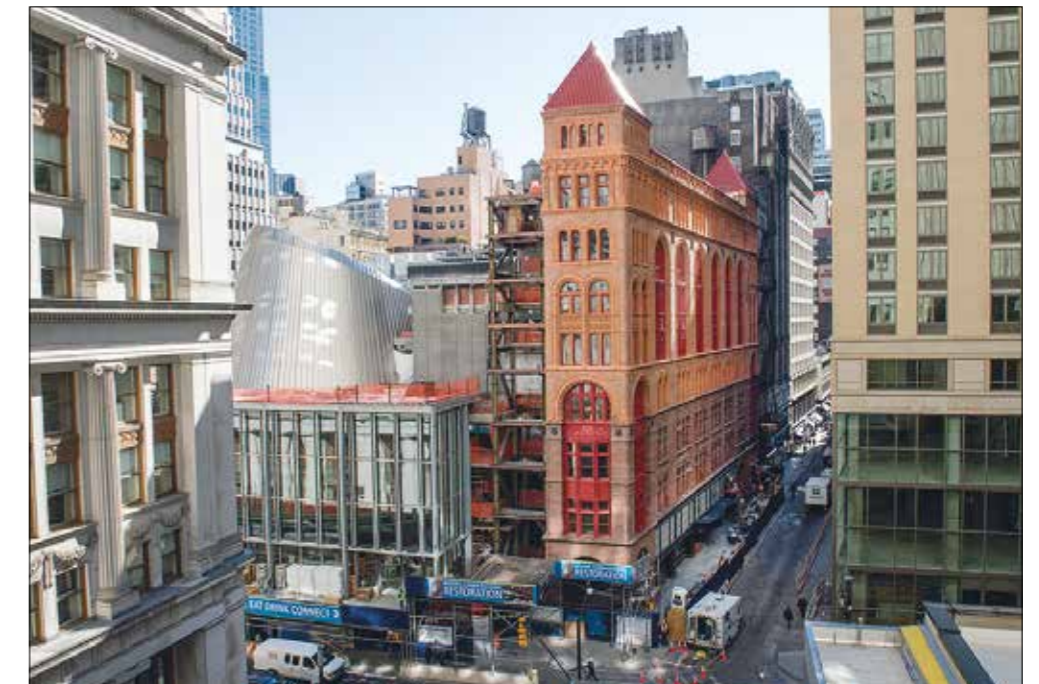
Looking across Broadway at the narrow west elevation of the Corbin Building, and the dome with its inclined oculus and skylight under construction to the north © Arup
