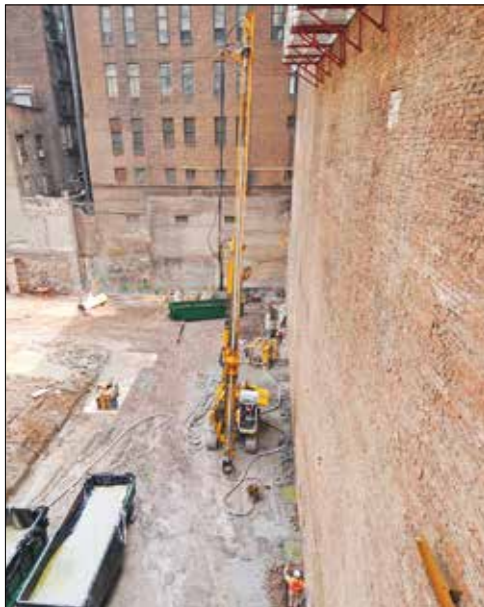
A jet-grouting rig stabilising the moving ground beneath the 'blind' north wall of the Corbin Building (on the right), to allow excavation to proceed below the building's foundations © Arup
