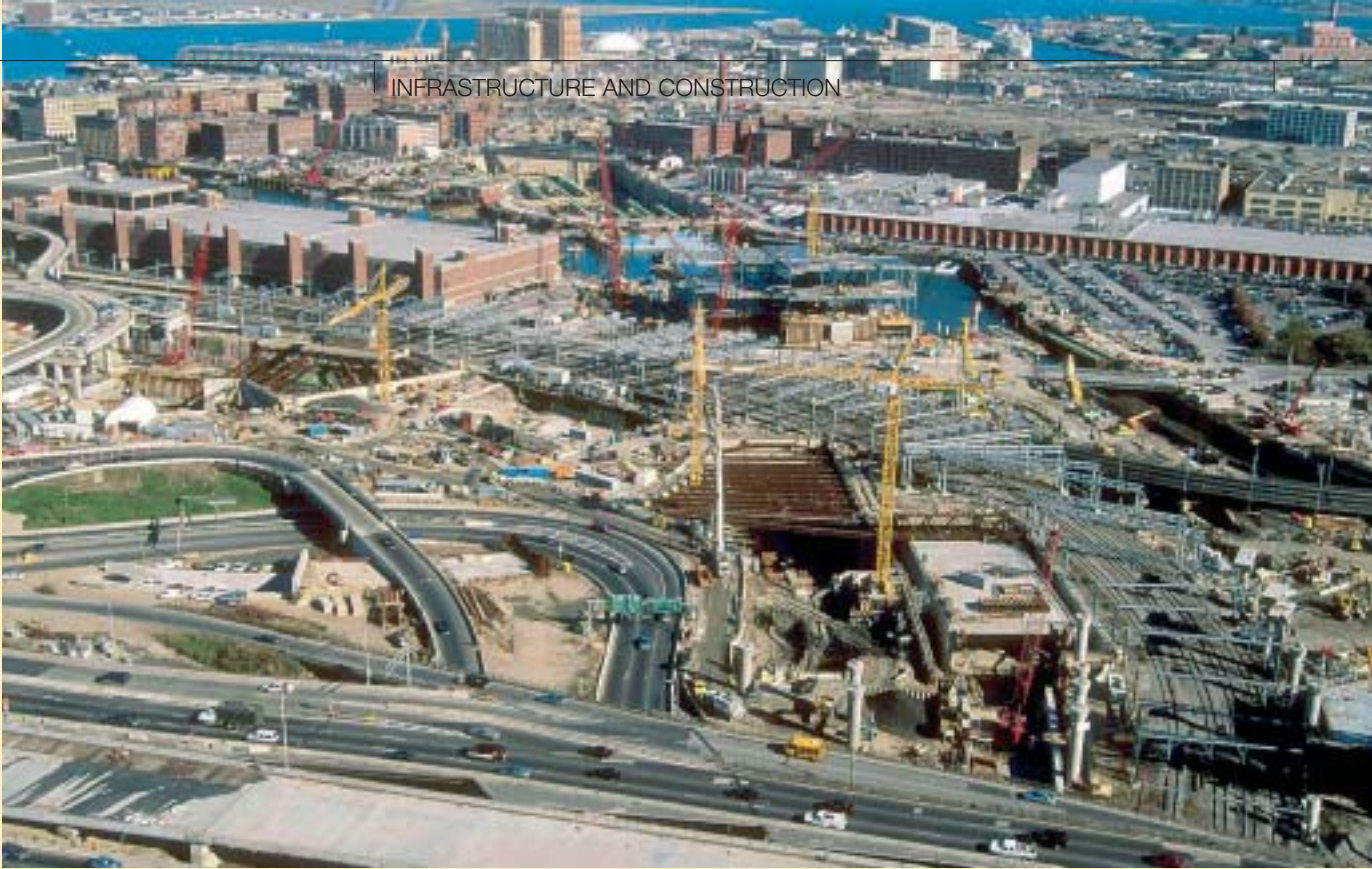
Figure 3 Site looking eastwards towards Logan International airport. The last unit of the I-90 jacked tunnel can be seen in the thrust pit on the lower right
