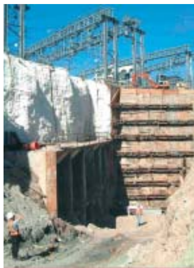
Figure 8 I-90 Westbound tunnel breakthrough on east side of railway. Jacked tunnel shield shown emerging below world's largest man-made iceberg
