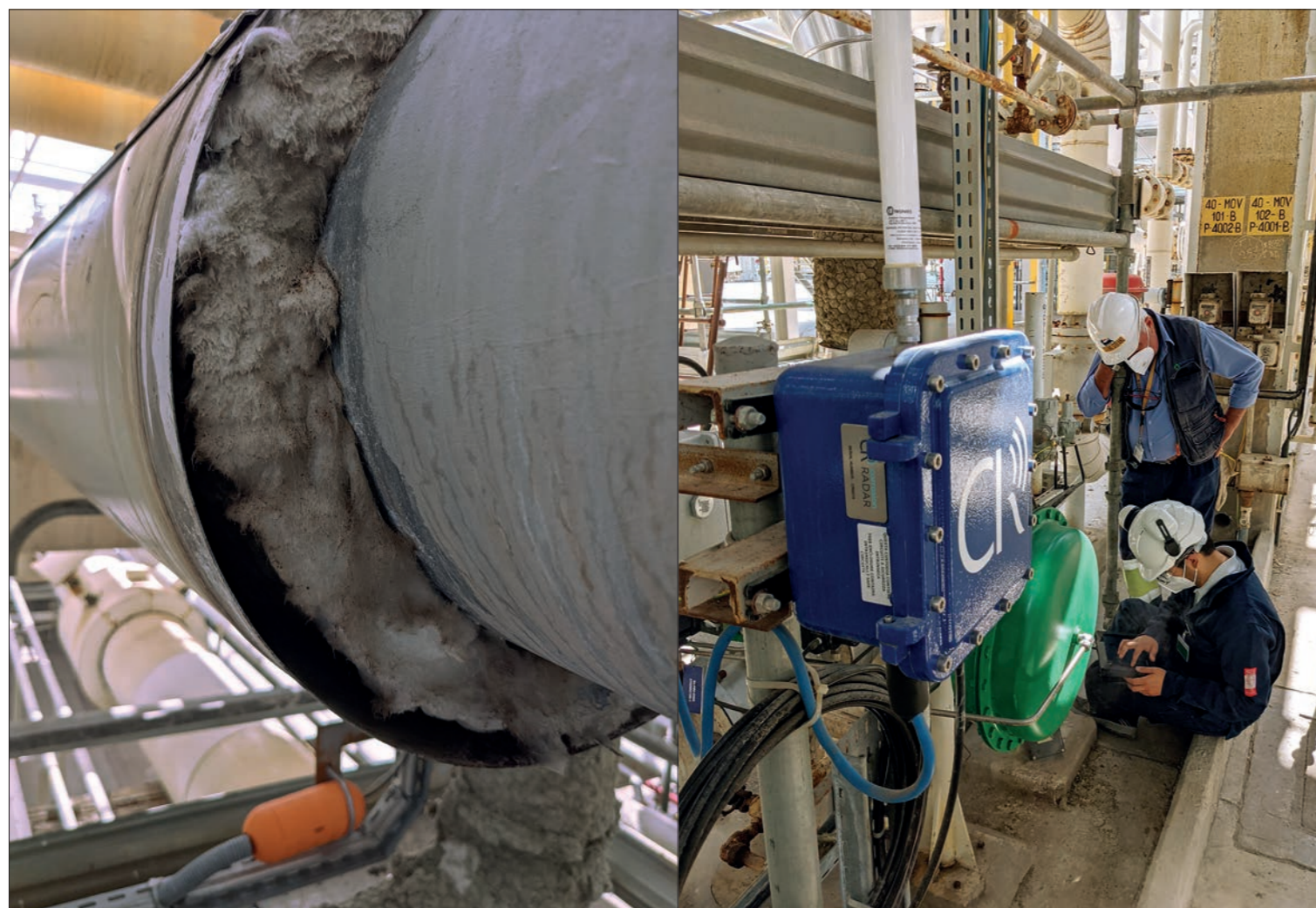
Left: Moisture sensors are fitted underneath insulation and metal cladding. Right: A control box that sends data from connected sensors to plant workers © CorrosionRADAR
