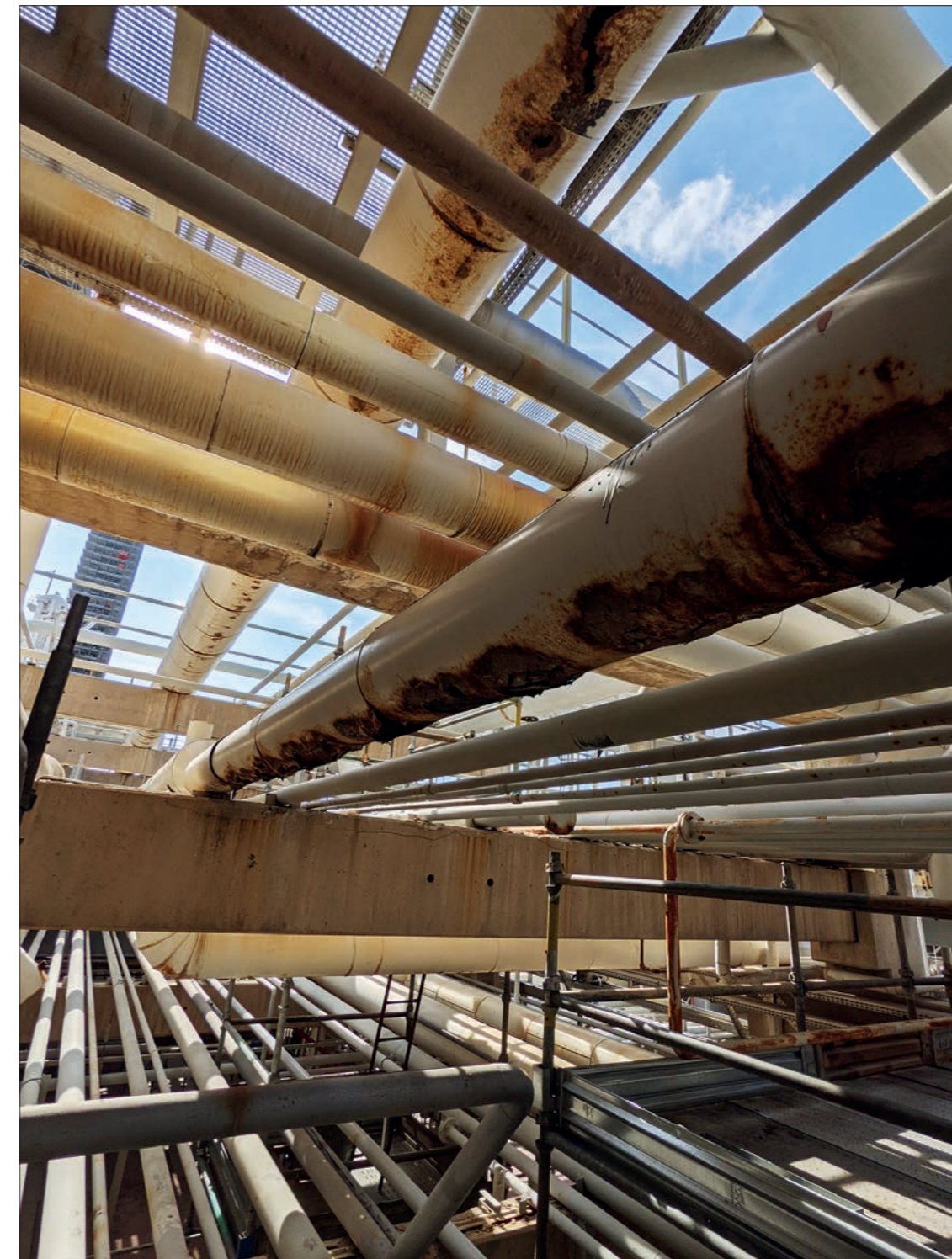
Pipe work at refineries is one of the places badly affected by corrosion under insulation. It can become visible at the bottom surface of pipes, where moisture is most likely to accumulate
