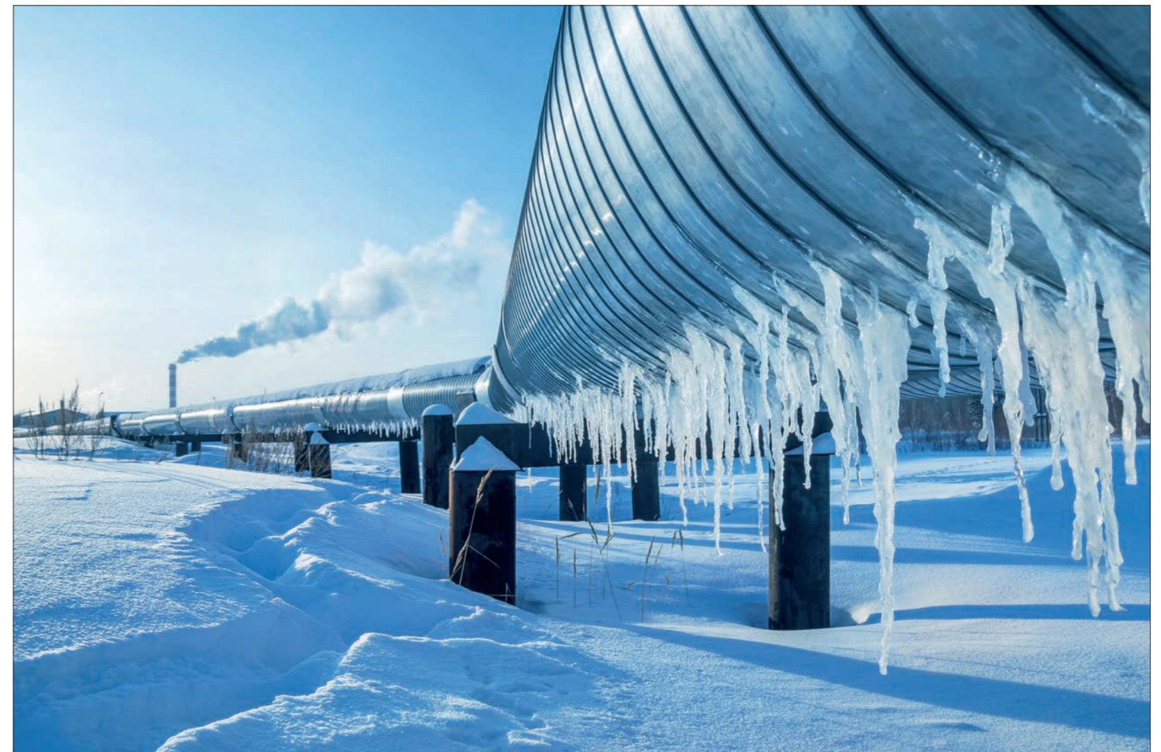
Pipelines are at the mercy of the elements, which fast-track corrosion. If allowed to gain a foothold, corrosion can cause chemical spills that devastate their surroundings © Leonid Ikan/iStockphoto
