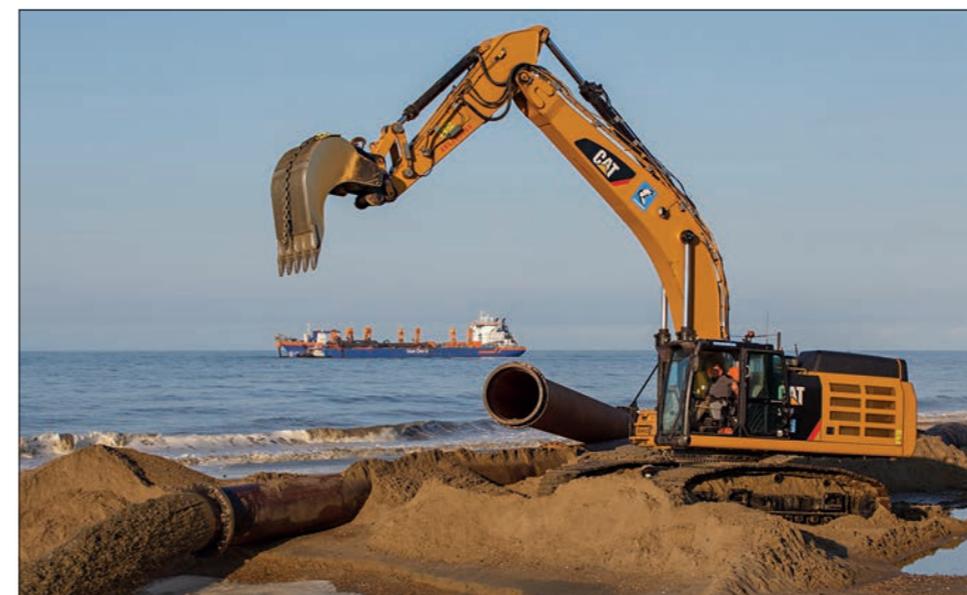
Contractors depositing sand for the mega nourishment at the beaches flanked by Bacton, Walcott, and the Bacton Gas Terminal © christaylorphoto.co.uk
