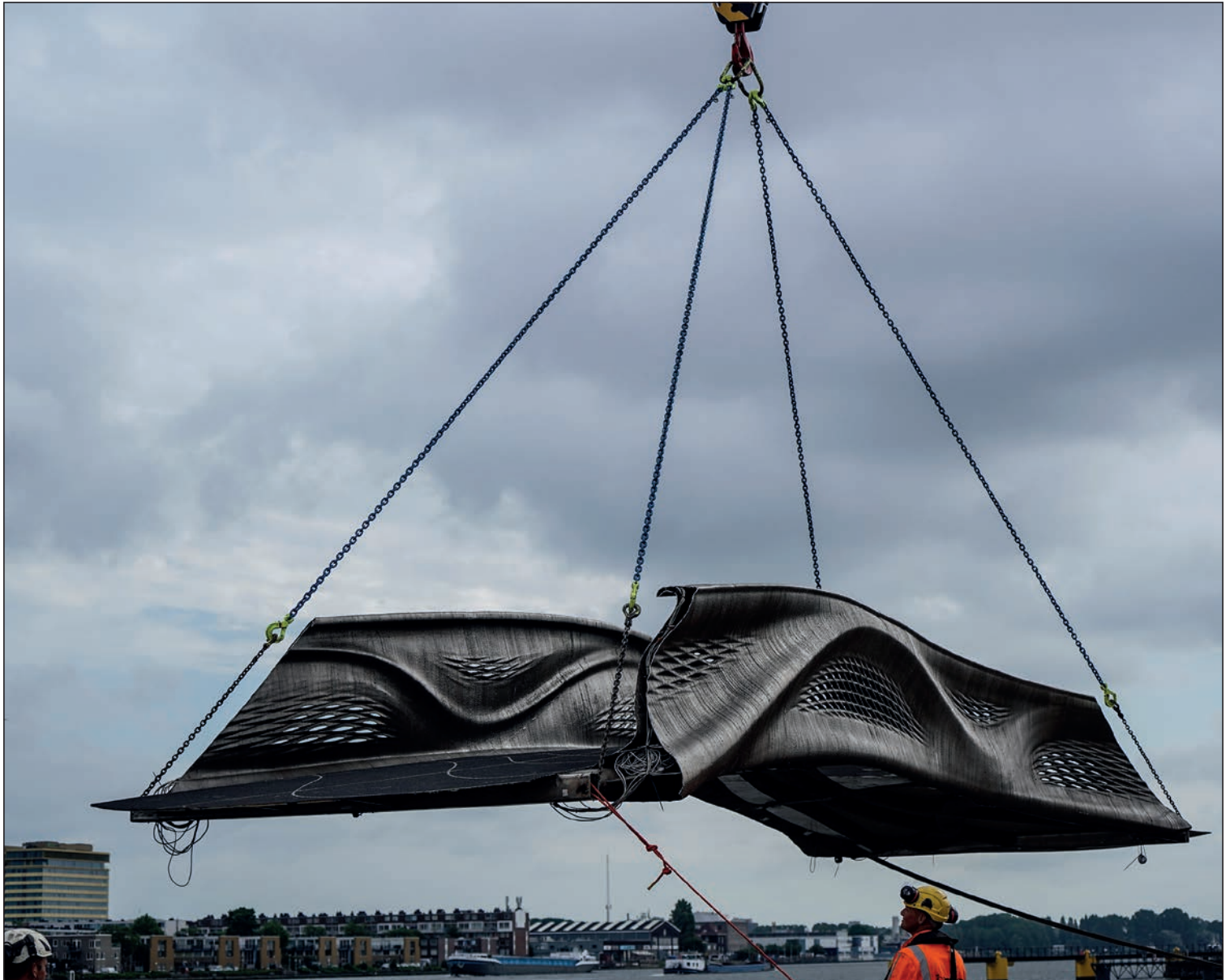
The central structural section of the bridge being transported to its final location © Merlin Moritz
