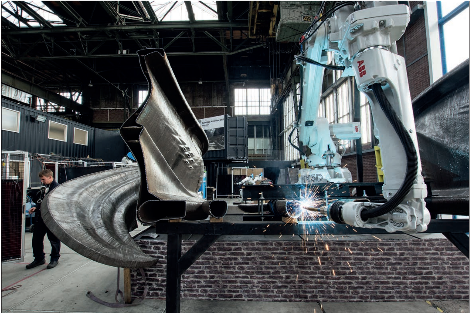
Printing of the bridge underway at MX3D's workshop in Amsterdam © Olivier de Gruijter
