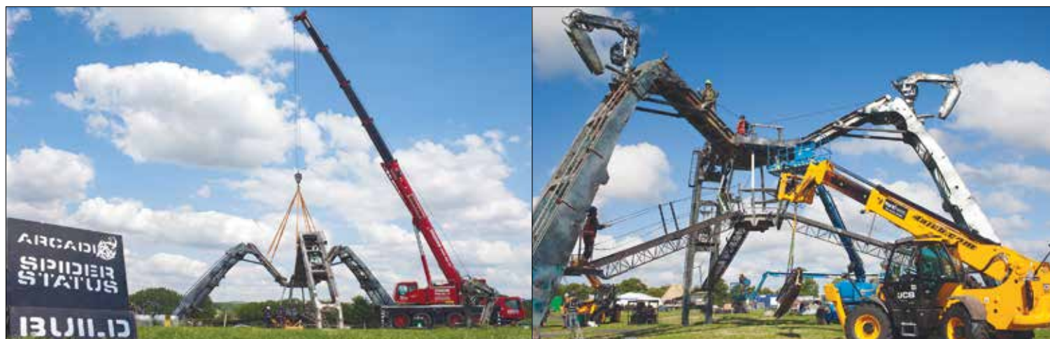
After the legs are attached to the Spider's main body, a crane lifts them up so that they pivot and stabilise the structure (left). Ancillary components are attached using hydraulic platforms (right) © Giles Mayall
